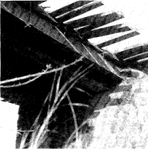
Partial destruction of wooden bridge deck.
