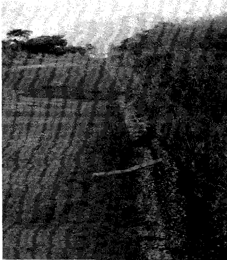
Rising shoulder due to spreading vegetation with localised road surface bumps.
