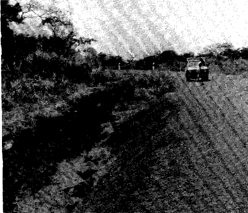
Regressive erosion of a side drain.
