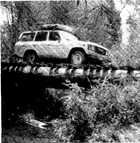
Accumulation of debris and vegetation below a bridge.
