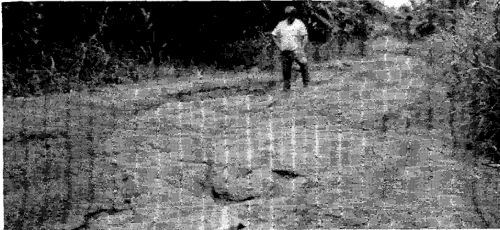
Longitudinal erosion gullies.
