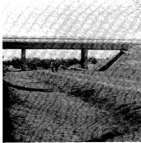
Erosion of shoulder and embankment
