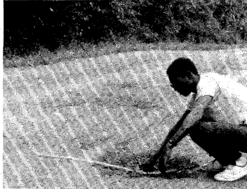
Pothole on dry roadway.
