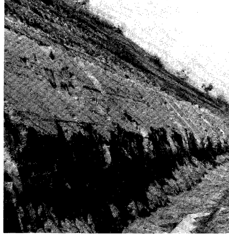
Slope erosion resulting in ditch siltation.
