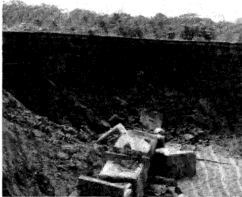
Total destruction of a gully with collapse of the pavement
