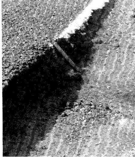
Lowered shoulder due to erosion. Starting deformation of road surface edges.
