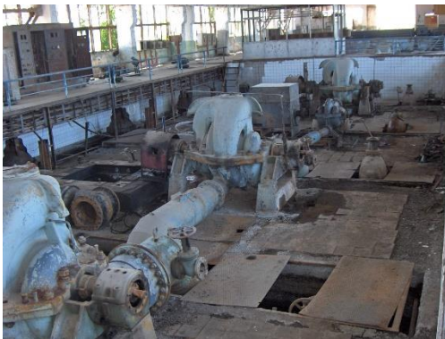
Fig. 3 Masis Pumping Station
