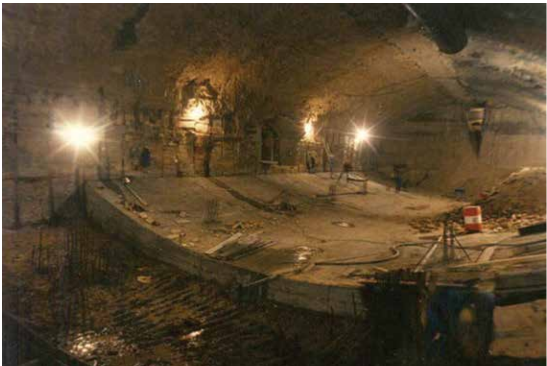
IMAGE 11.3. Construction of a Station Using the German Method along Metro Line 6: Madrid, Spain
