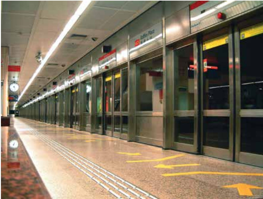
IMAGE 5.2. Full-Height Platform Screen Doors: Raffles Place Station, Singapore
