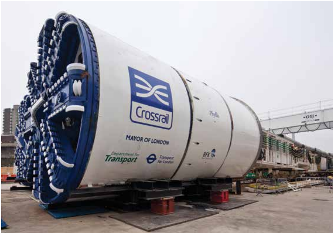
IMAGE 11.5. One of Crossrail’s Tunnel Boring Machines, with Back-End Supply of Power, Water, and Concrete Segments
