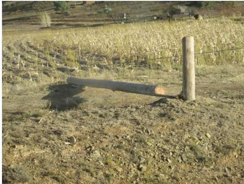
Figure 23: ETL pole on route to Mohale's Hoek which was cut down by thieves or vandals
