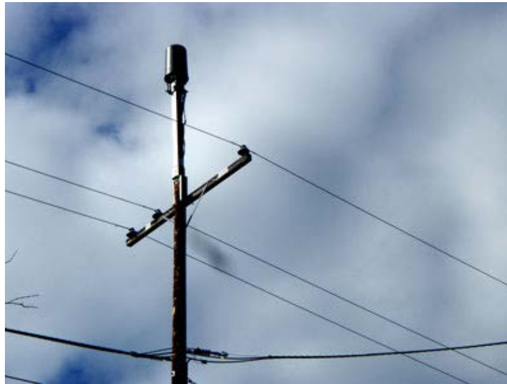
Figure 8.14: AT&T distributed antenna system installed atop electricity distribution pole in California
