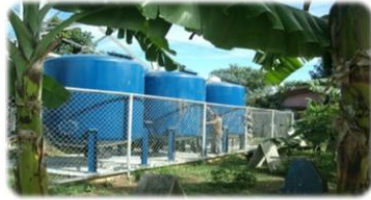
Installed advance water filtration systems
